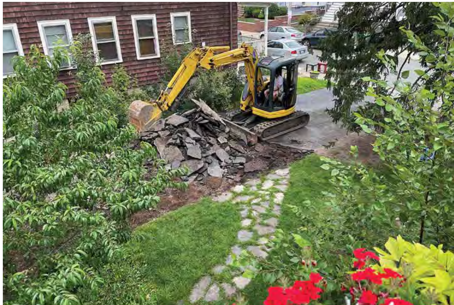
The driveway came out without a fight! The ledge we discovered beneath it, however, was another story and required a creative workaround.
